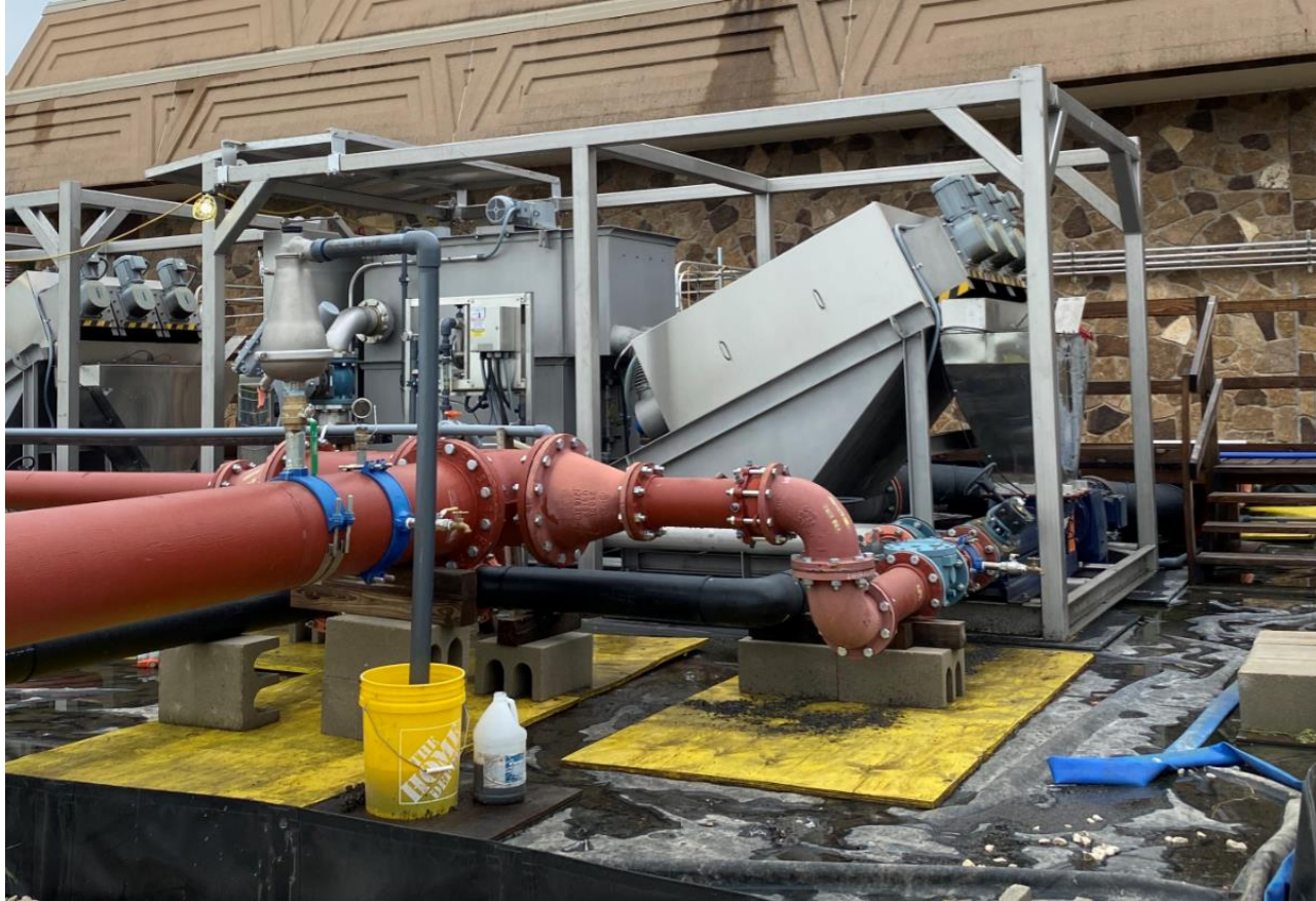
Temp. Facility - Walnut Creek WWTP
